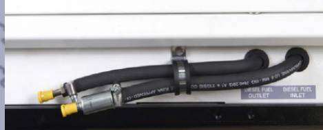
INPUT/OUTPUT FUEL PIPE
