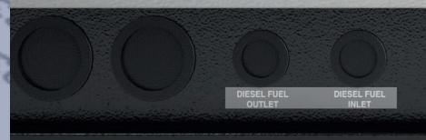
INPUT/OUTPUT FUEL PIPE
