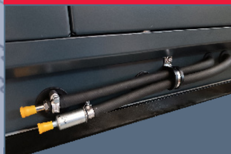
INPUT/OUTPUT FUEL PIPE
