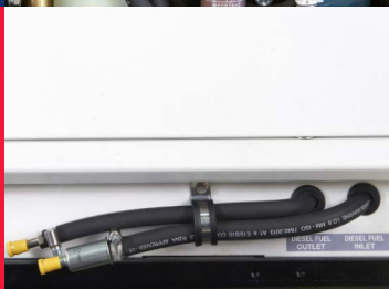
Input/Output fuel pipe
