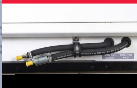
INPUT/OUTPUT FUEL PIPE
