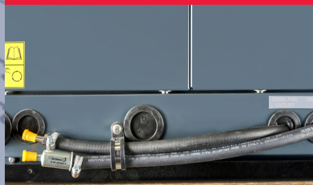
INPUT/OUTPUT FUEL PIPE
