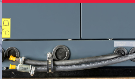
INPUT/OUTPUT FUEL PIPE
