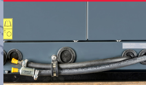
INPUT/OUTPUT FUEL PIPE
