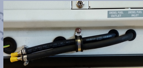
INPUT/OUTPUT FUEL PIPE
