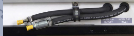
INPUT/OUTPUT FUEL PIPE
