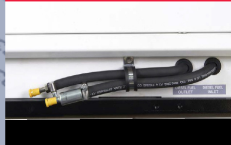
INPUT/OUTPUT FUEL PIPE
